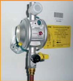
Typical Truma regulator installation mounted vertically. The 10mm copper compression fitting has been unscrewed for changing.
